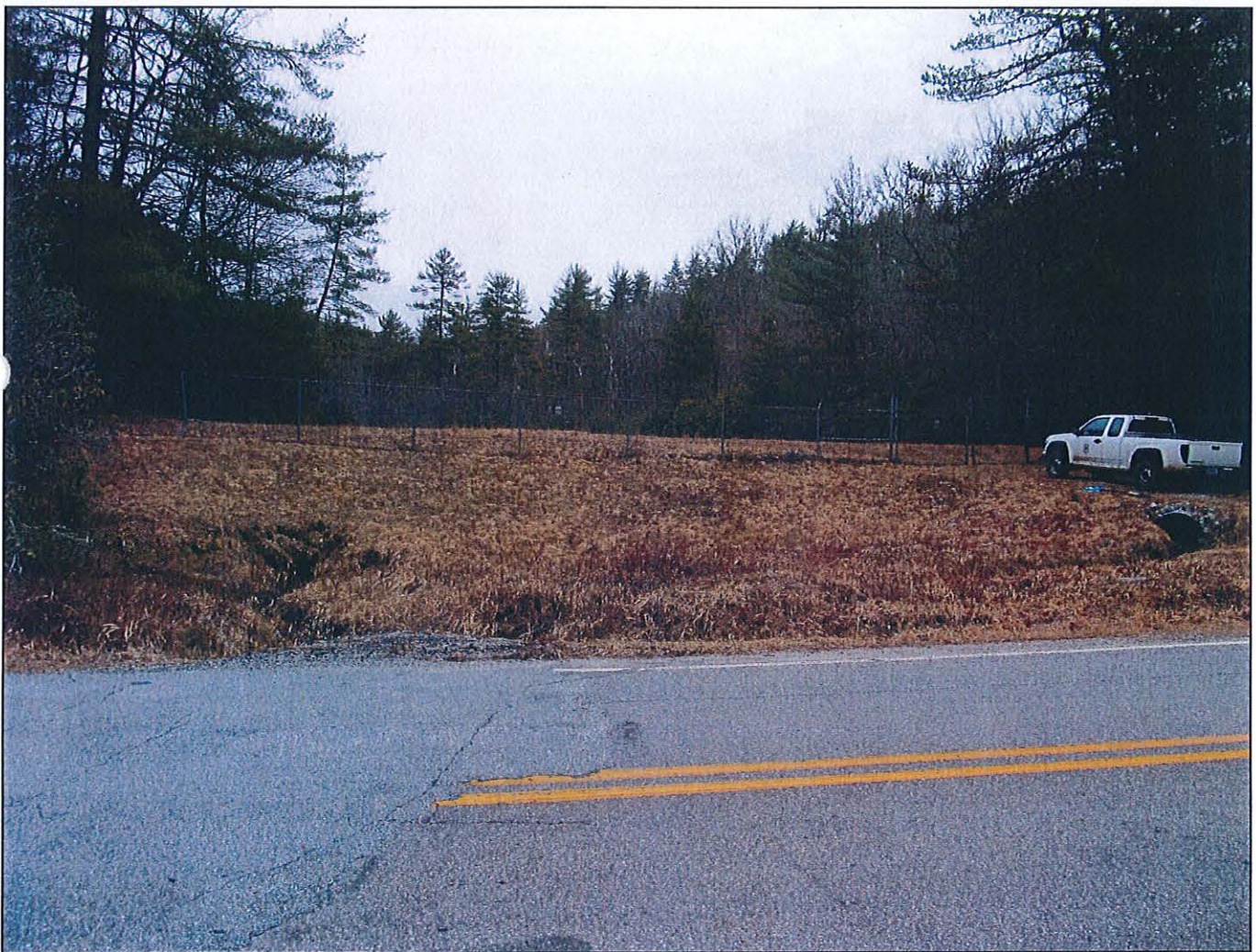
Plate 1. View north, showing the 12-foot tall earthen Houston Dam at Highlands Reservoir. North Carolina State Highway 1538 is in the foreground. Note eroding face of the dam in left foreground.
